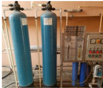
DRINKING WATER TREATMENT PLANT
