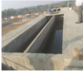
STP PLANT - WASTE WATER TREATMENT
