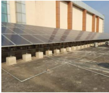
ROOF TOP SOLAR POWER PLANT
